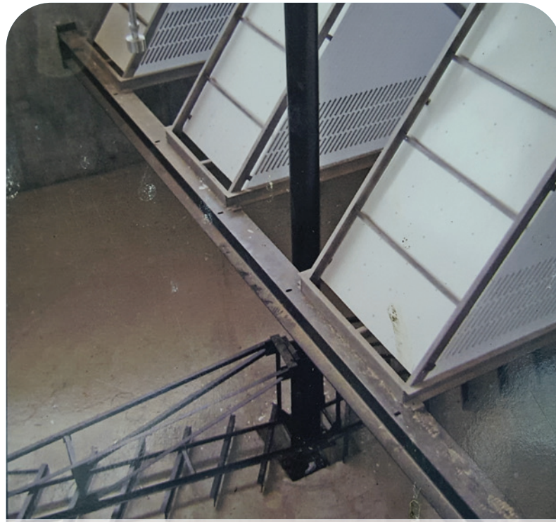
Plate pack and sludge rake mechanism
