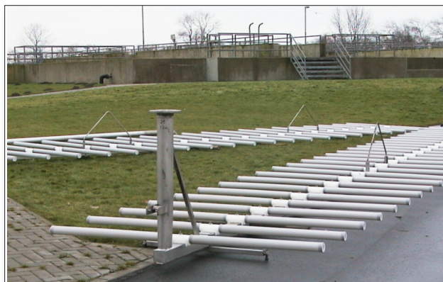
The grids equipped with OTT System MAGNUM 2000 FLEXSIL HE® diffusers are ready to be re-installed.
