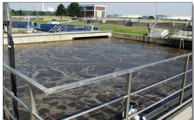
The bubble pattern is extremely fine and uniform after the rebuilding of the first line – a token of high-quality and efficient membrane diffusers.
