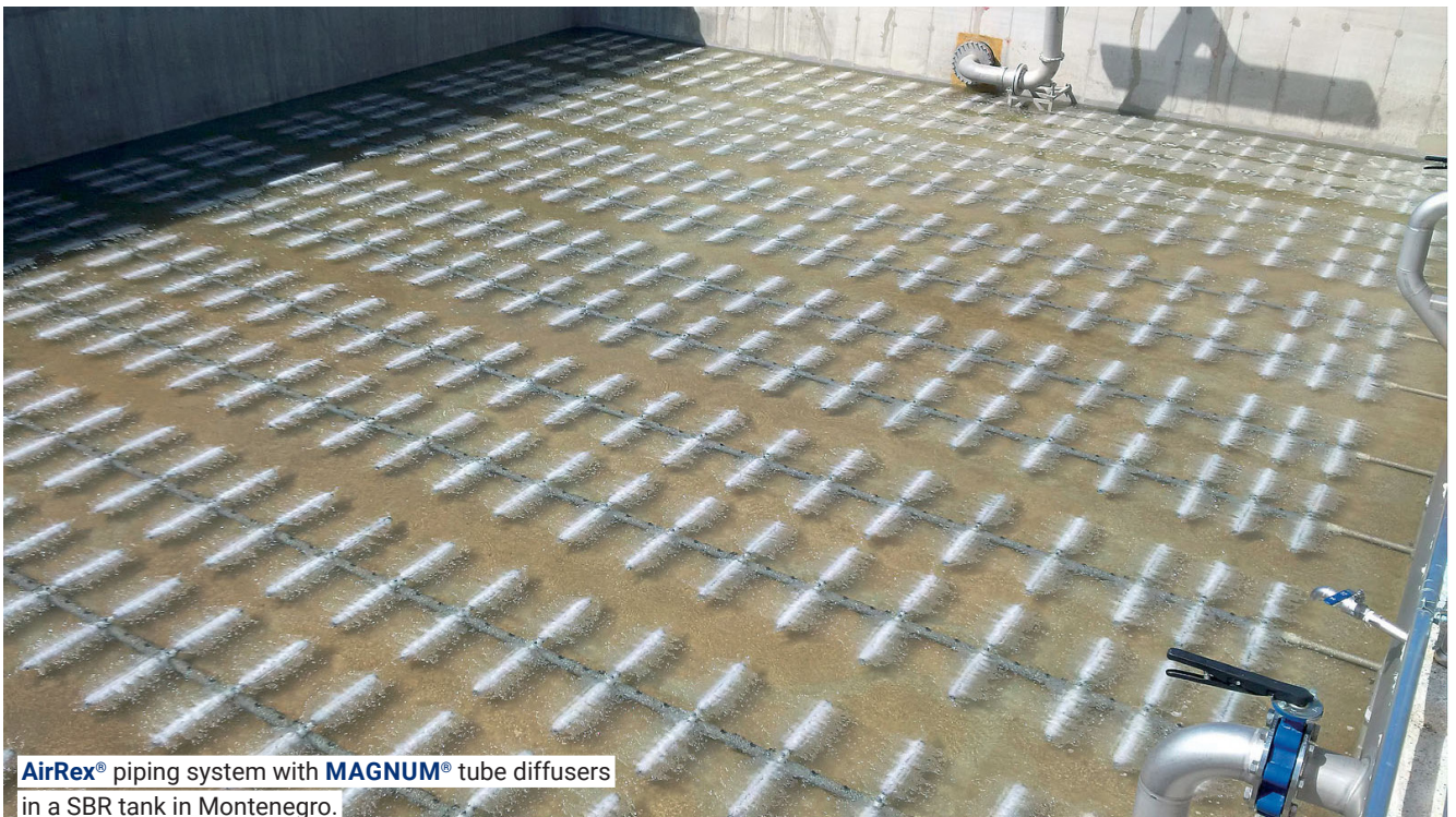
AirRex® piping system with MAGNUM® tube diffusers in a circular tank in Northern Germany
